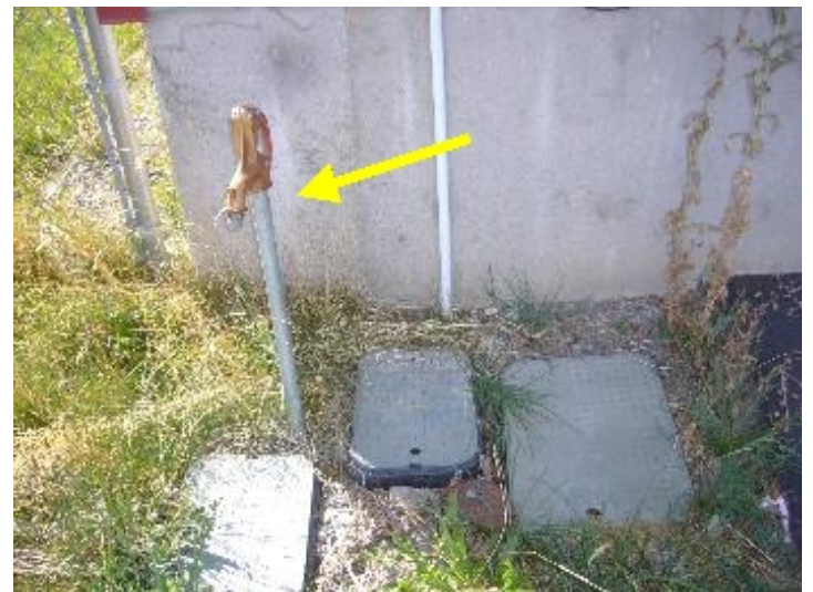
Water hydrant at right rear of building
