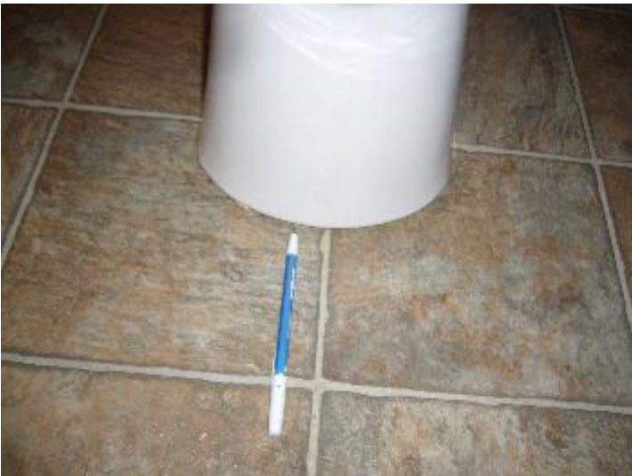
Caulk around toilet in office restroom
