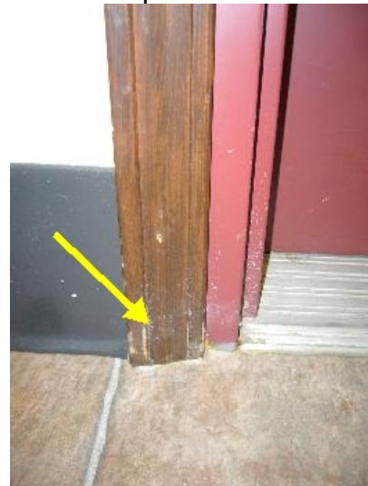
Some minor areas need prep, and paint or stain
