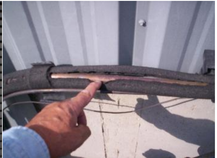
Damaged A/C Line set insulation
