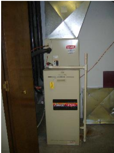
View of furnace
