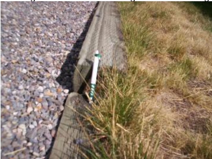
Potential trip hazard at RR ties at right side of building
