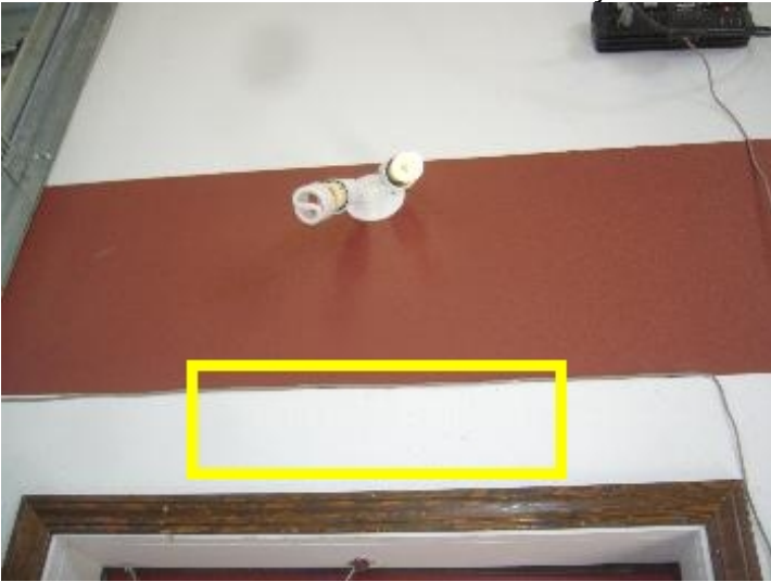
No Exit lights at exits
