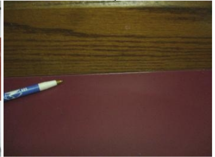
Minor caulk needed at kitchenette sink backsplash
