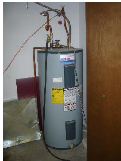
View of water heater
