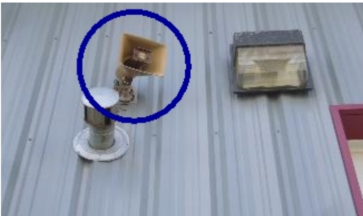
Speaker at rear wall on same line as garage heater
