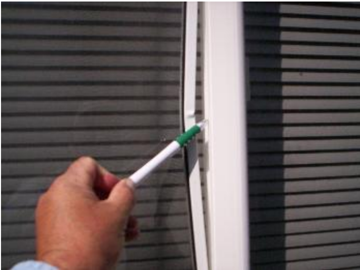
Damaged window screen at right side of building
