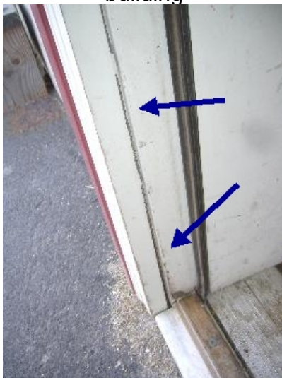
Rear door frame slightly loose
