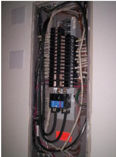
View of electrical panel box
