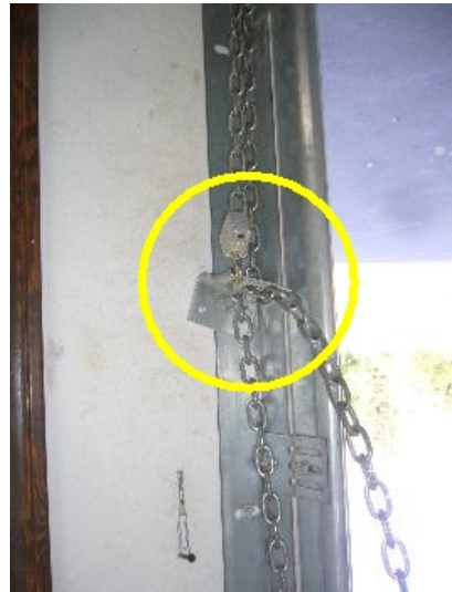
Keep pull chain for rear garage door secured
