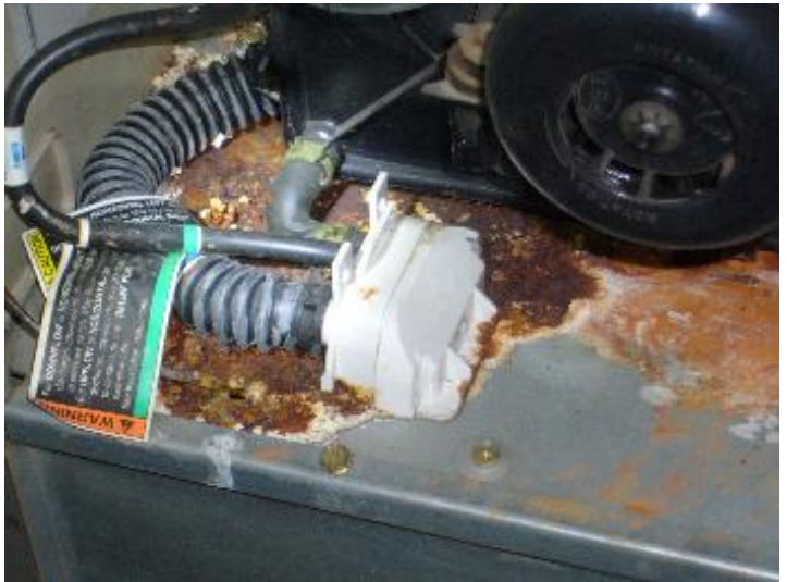
Corrosion inside furnace
