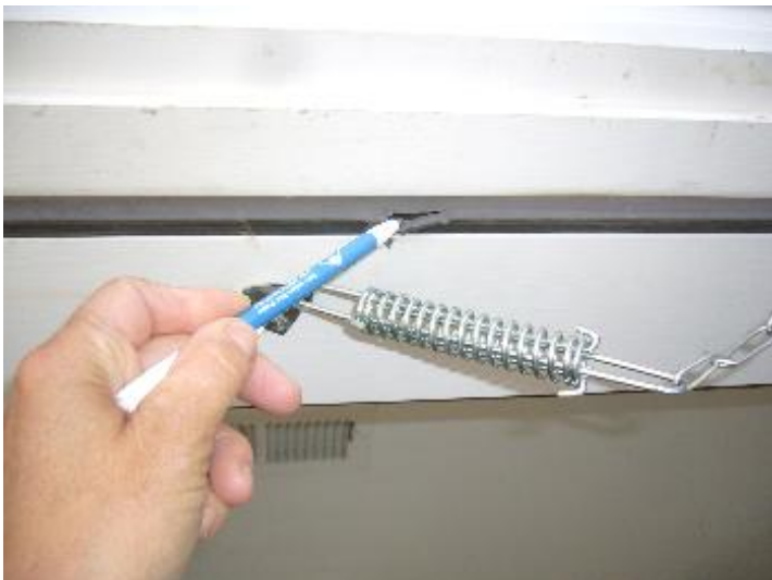
Minor damage to front door weather strip
