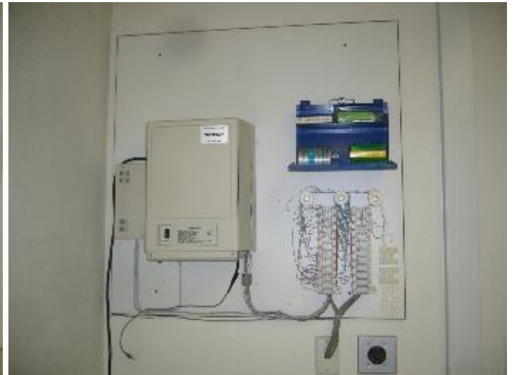
Telecommunications system & first aid kit
