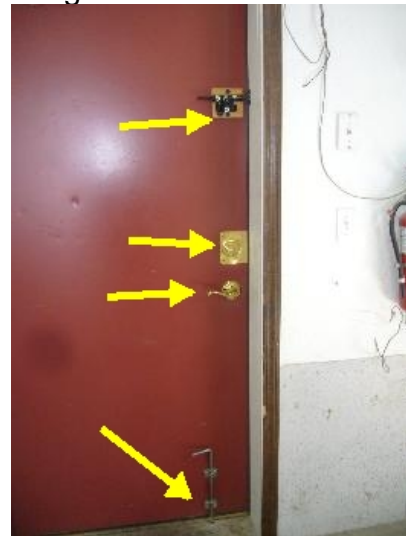
Several Locks at rear door
