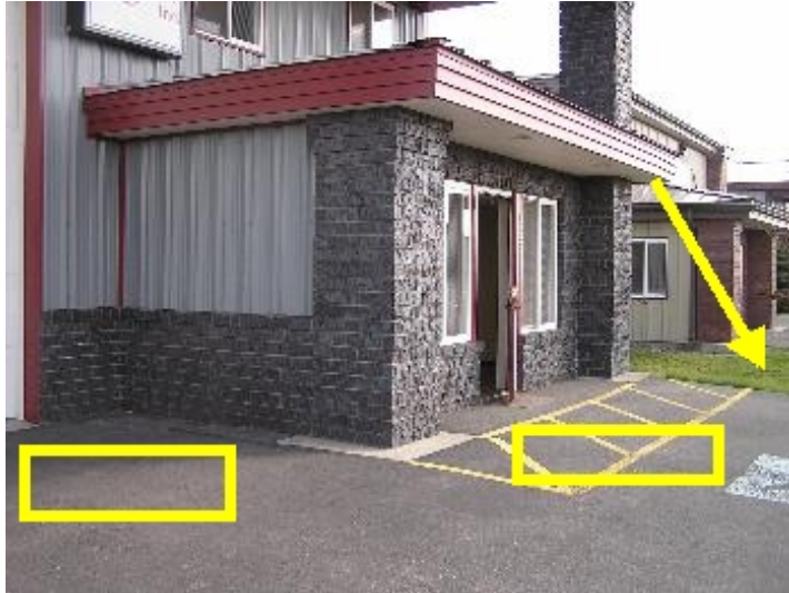
Consider system to carry water from entranceways
