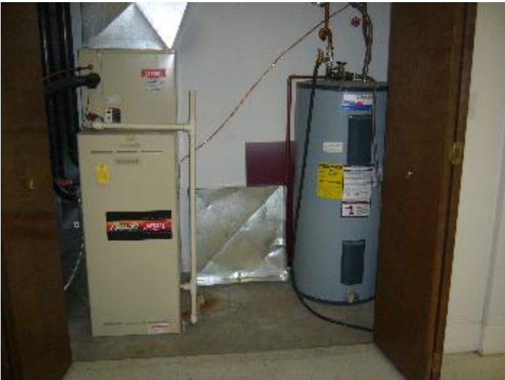
Furnace & hot water heater in utility closet
