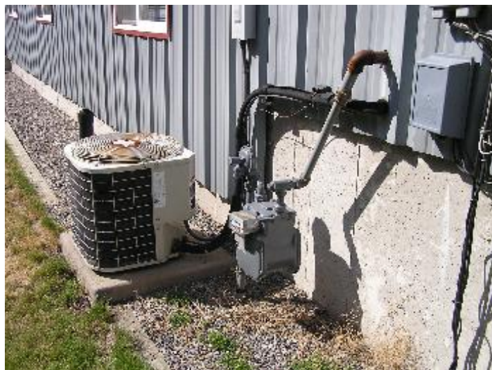
View of A/C unit at right side of building
