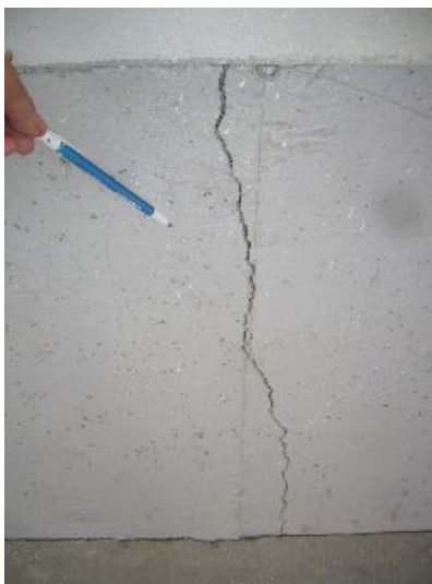
Normal settlement cracks noted
