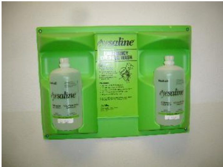
Eye wash located in restroom off garage
