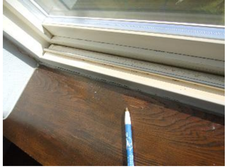
Evidence of minor condensation at right side windows
