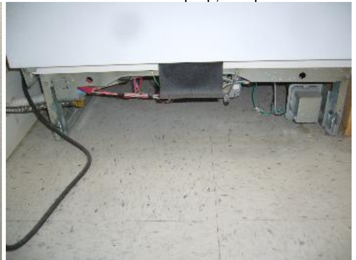
Bottom cover missing at dishwasher
