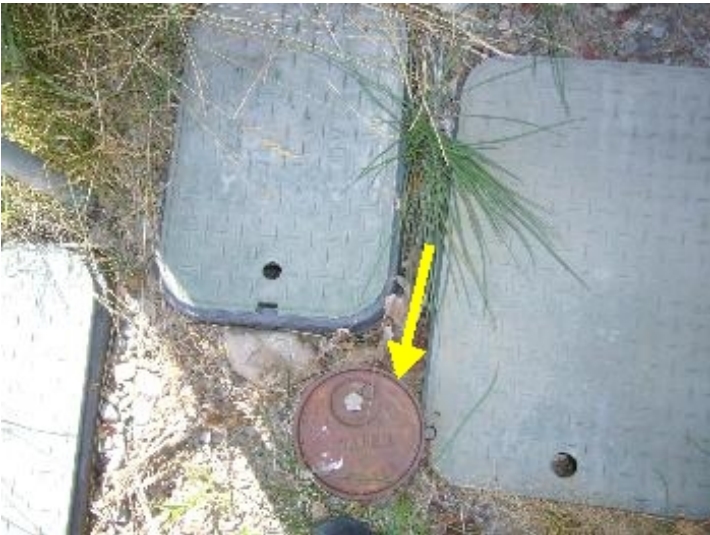
Water meter at right rear of building
