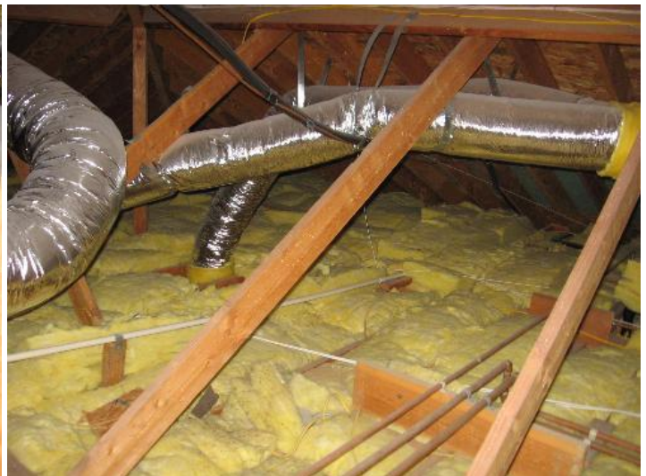
Attic Duct Work
