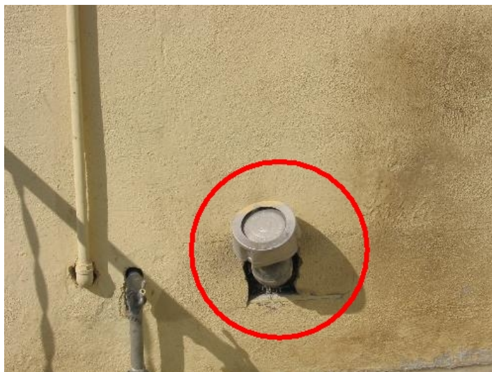
Improper installation of vent pipe. Exhaust vent from water heating in the basement area.
