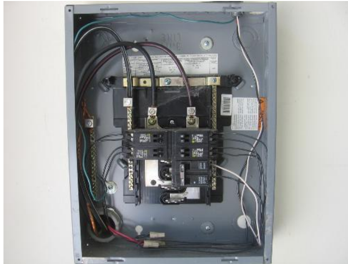
Electrical Sub Panel
