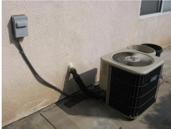
Heating AC Compress Condition
