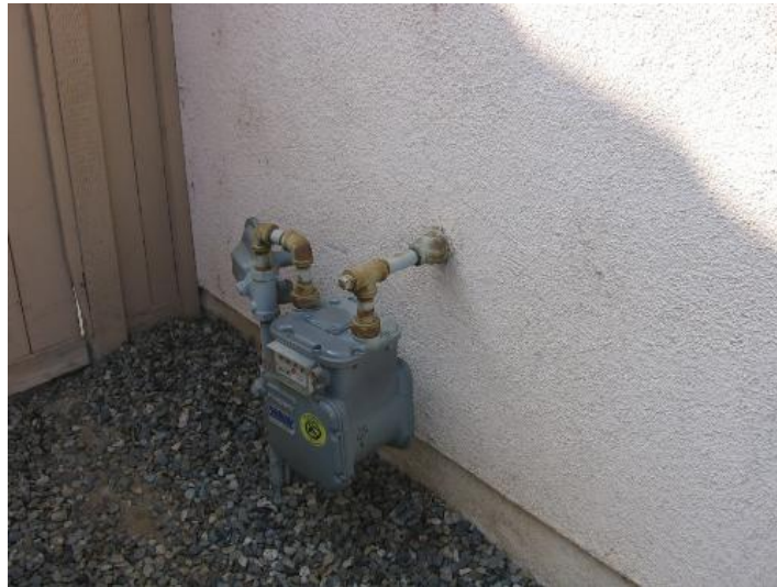
Main Gas Valve
