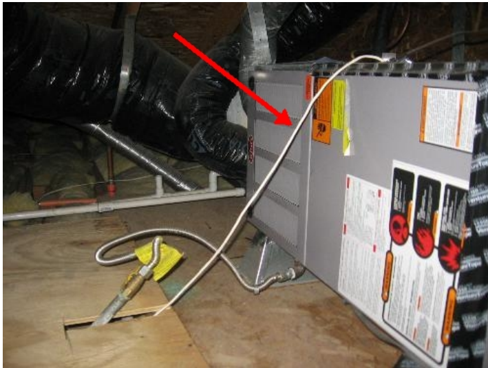
Downstairs heater view.
