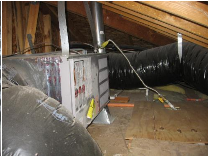
Heating Heater Condition
