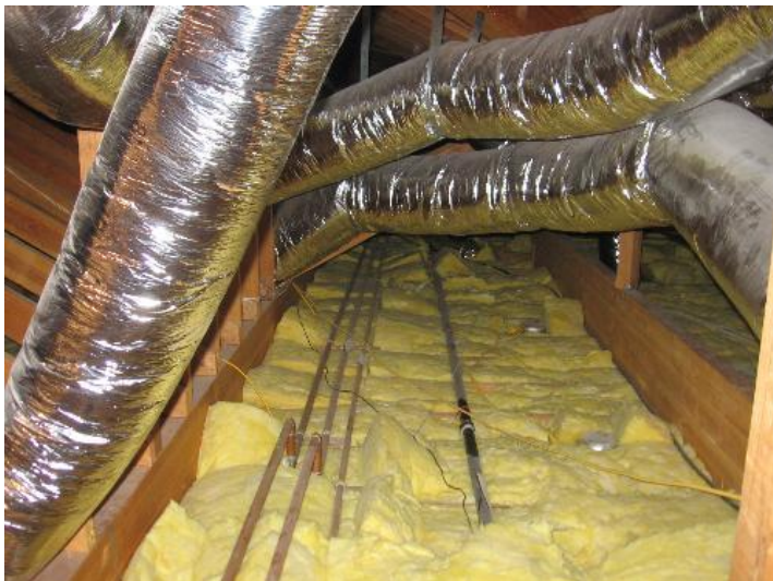
Attic Duct Work
