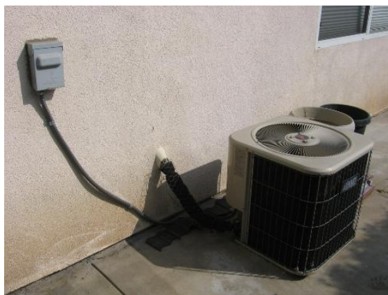
Heating - AC Compressor
