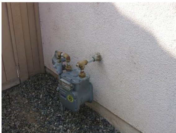
Exterior - Main Gas
