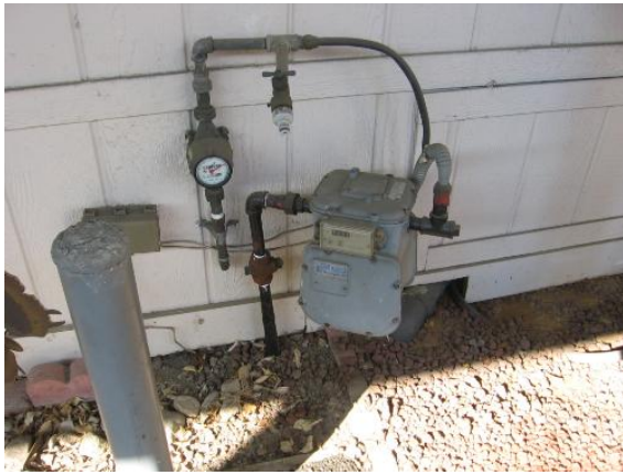
Exterior - Gas Meter
