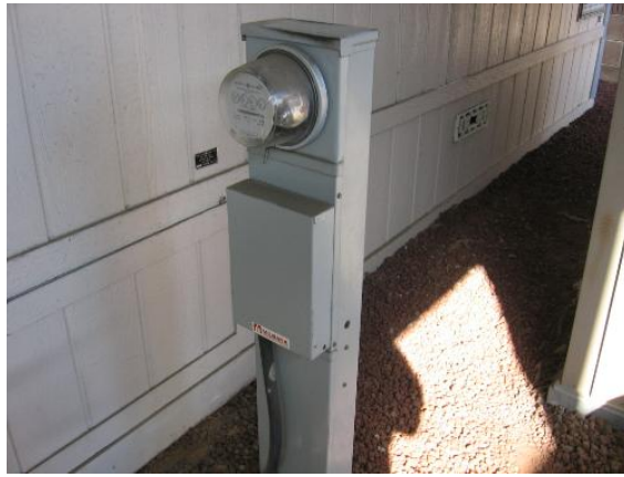
Electrical - Service Panel
