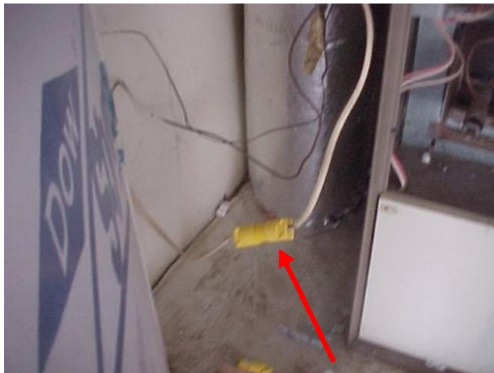
Improper electrical supply to furnace
