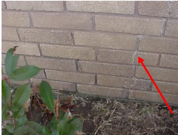
Hair line mortar joint crack below window west side S.W. corner
