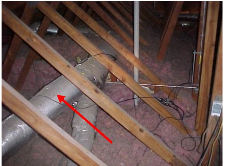
A/C ducts in the attic same as Infrared Picture
