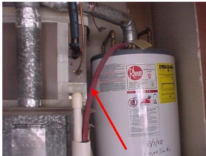
Improper Relief valve downspout hot water heater
