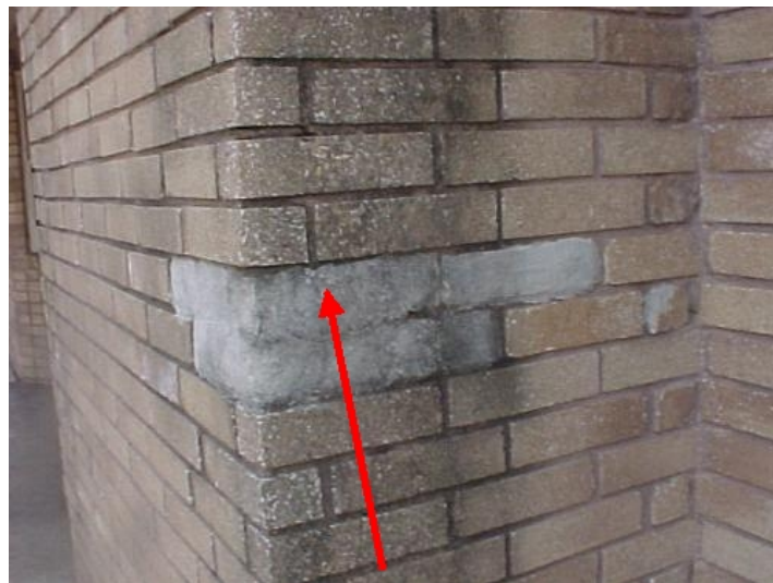
Cosmetic brick spalling exterior chimney as the result of no guttering
