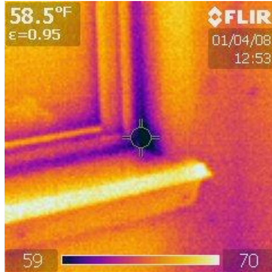
Infrared image indicating air intrusion at the corner of the windows dining room
