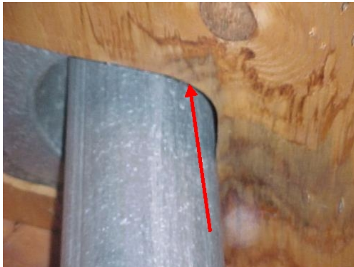
Furnace flue vent improper clearance at the roof
