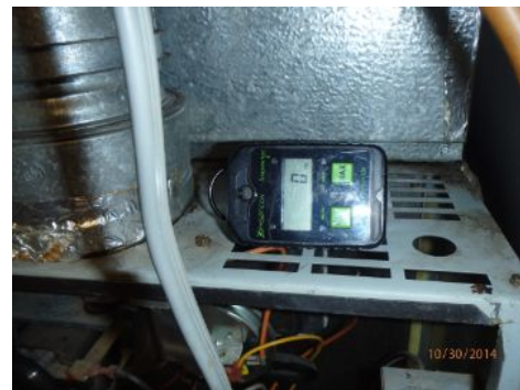
Co2 levels normal around furnace
