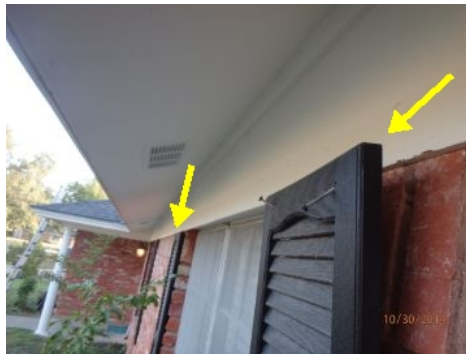
Window shutters on exterior side of home was loose at top and not secured to brick wall,
