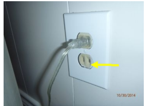
All of the two prong outlets and most of the three prong outlets are on a two wire system with no ground.
