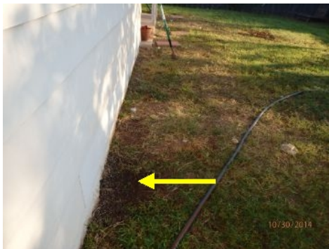
Signs of poor drainage at back side of home. Large holes against foundation should be filled to allow water to drain away from foundation.
