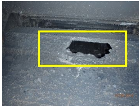
Large hole inside of firebox near dampener.
