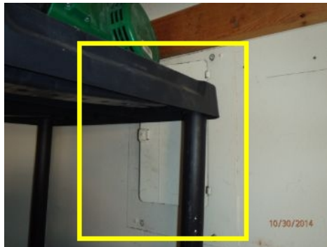
Could not open and inspect inside of panel box due to personal items and shelving blocking door.
