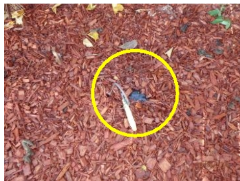
Sprinkler head in back yard was located under weed barrier.
