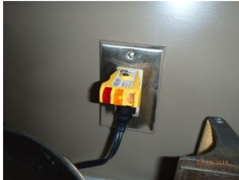
Open ground on kitchen GFCI
