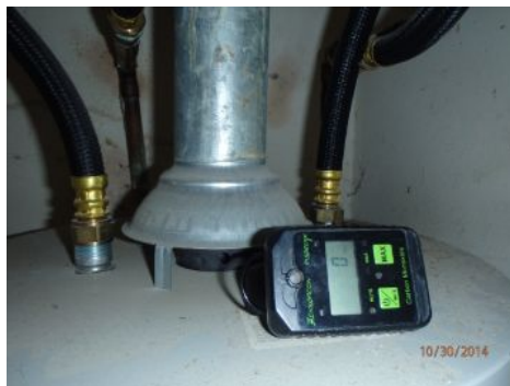
Co2 levels were normal around water heater
