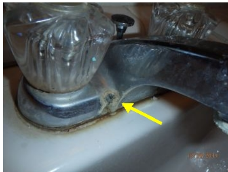
Corrosion present around bathroom valve. No leaks from this spot at time of inspection. See picture
