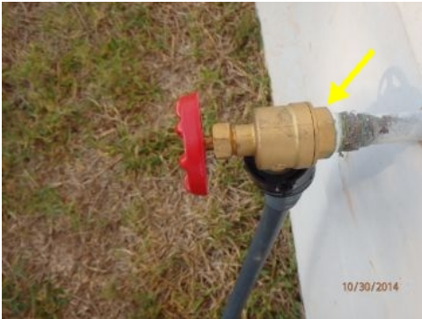
Hose bib needs to be tightened at back of home. No leaking at time of inspection.
