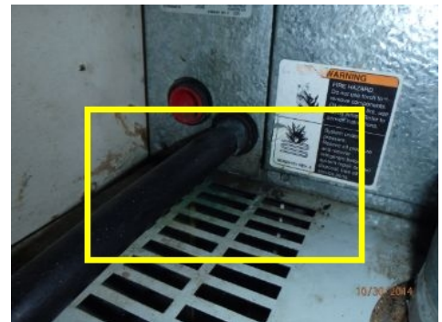
Evidence of past leaks from unit near condensate drain line and flooring around unit. No evidence of any leaks at time of inspection.
