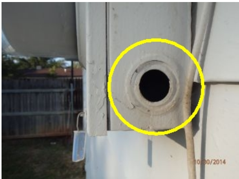
Knockout needs snap-in cap at meter box at exterior.
