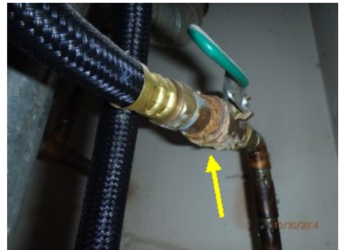
Corrosion present around shut off for water heater
