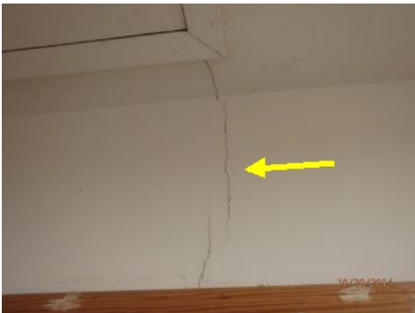
Settlement cracks were observed at various locations. Cosmetic damage was observed.
