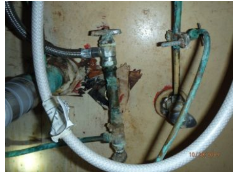
Corrosion present around valves. No evidence of any leaks
