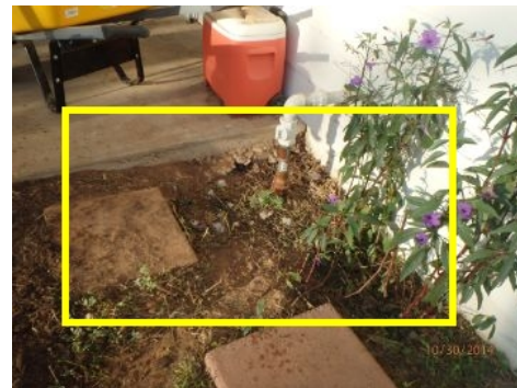
Large hole against foundation at back of home
