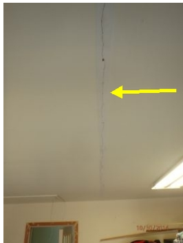
Small cracks on ceiling in garage hallways. Cosmetic
