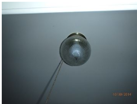
Light fixture inoperative at time of inspection. Possible spent bulb. Closet
