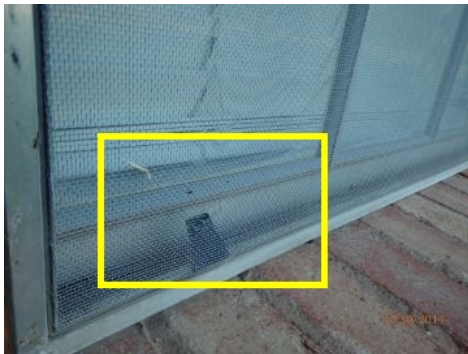
Small hole in screen on window at front of home.
