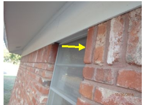
Loose brick on south side of home left of garage door. This is not a structural issue. Cosmetic
