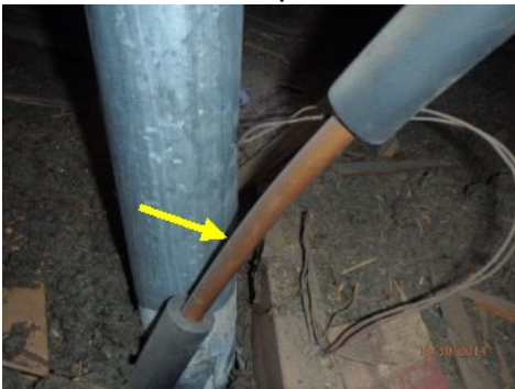
Supply line from water heater to bathroom has been replaced at some point in attic. Some of the copper pipe in attic has had insulation placed over it. There are two spots missing insulation that should have it.
