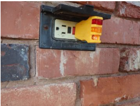
Exterior plugs were not grounded
