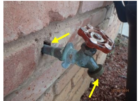
Exterior hose faucets do not have back flow protectors. Recommend sealing hole around hose bib
