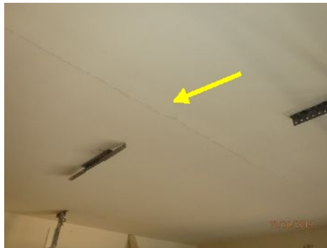
Cracks on ceiling in garage, Cosmetic
