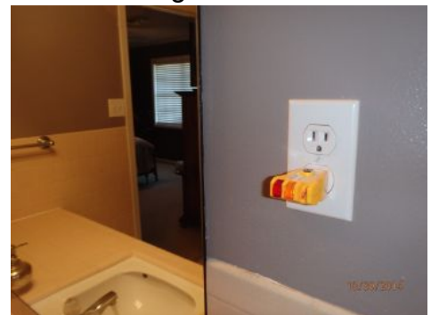
No GFCI on bathroom receptacle
