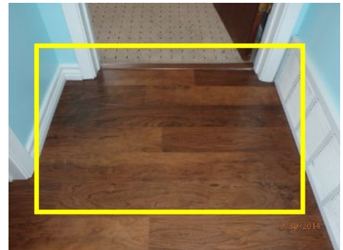
The floor adjacent to the HVAC closet shows evidence of water damage. It appears that A/C may have leaked at some point onto wood laminate flooring. No leaks from this area at time of inspection
