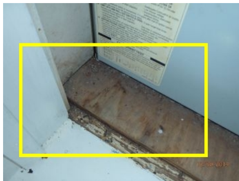
Evidence of past leaks under HVAC closet
