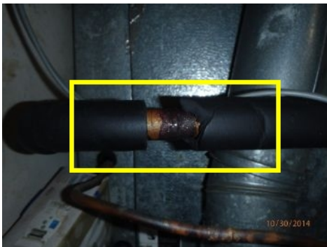
Refrigerant line was not fully insulated at the unit. This condition causes the line to sweat and slightly degrades the performance of the system.
