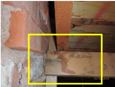
Area inside of attic around chimney shows evidence of past leaks. Also visible light was viewed from inside of attic.
