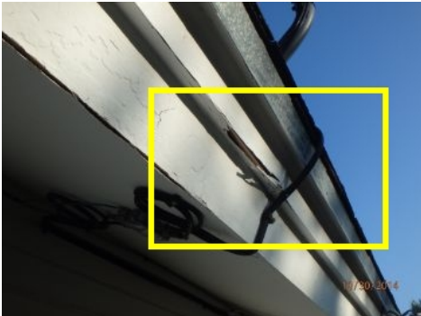
Small area on back eave has exposed. Wood should be painted before further damage.
