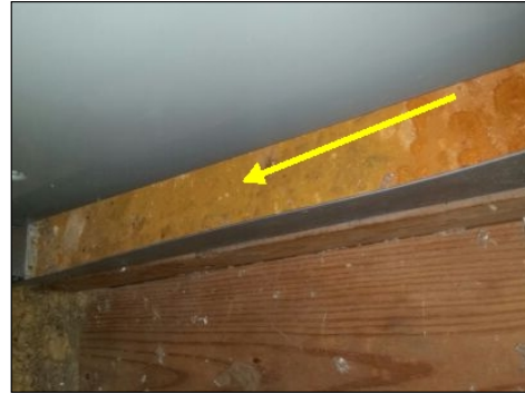
Rust in condensate pan
