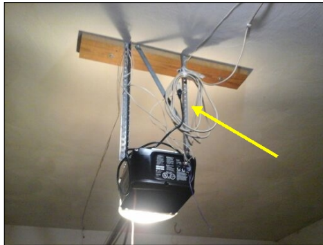
Extension cord wiring
