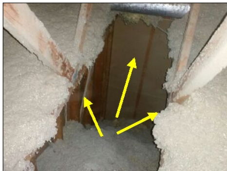
Areas missing insulation
