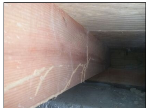
Termite tubes observed
