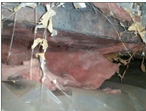
Insulation damaged at ductwork
