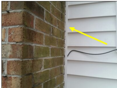
Sealant maintenance needed
