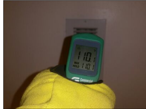
Auxiliary heat functional
