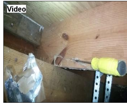
CLICK to VIEW video of crawlspace issues
