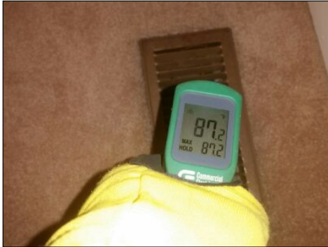
Auxiliary heat functional
