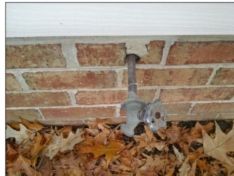
Loose hose bib
