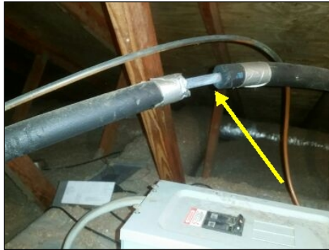
Repair or replace insulation
