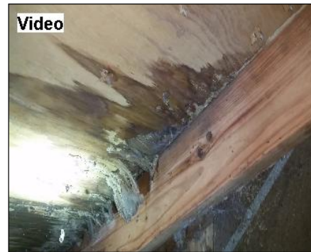
CLICK to VIEW video of garage attic damage
