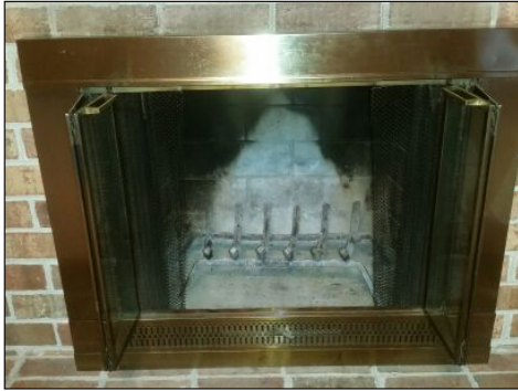
Masonry wood burning fireplace
