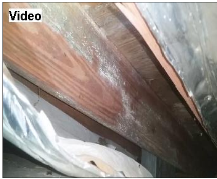
CLICK to VIEW video of crawlspace issues
