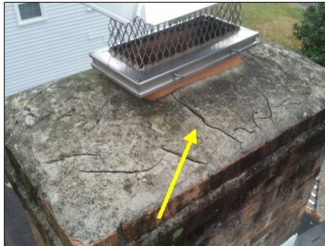
Chimney crown needs repair
