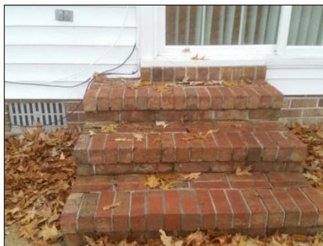
Uneven risers and no handrail
