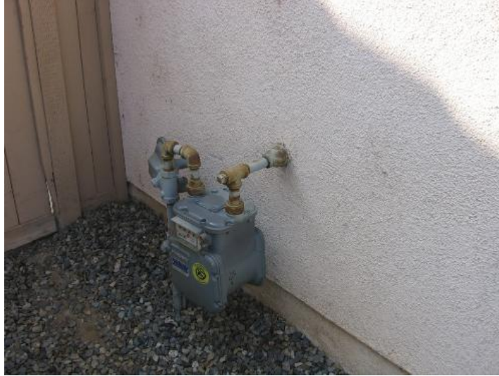
Main Gas Valve
