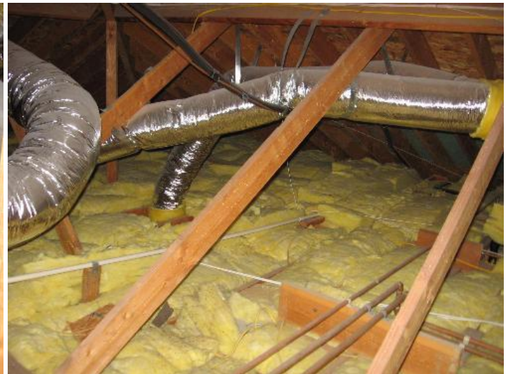
Attic Duct Work
