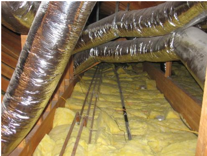
Attic Duct Work
