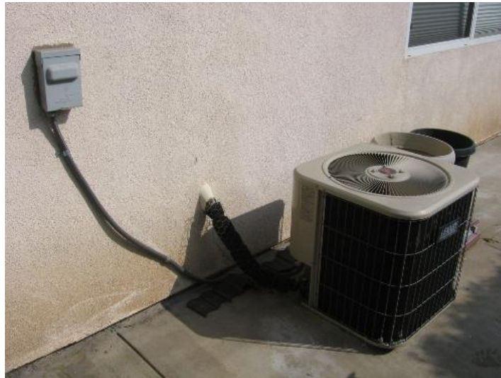
Heating AC Compress Condition
