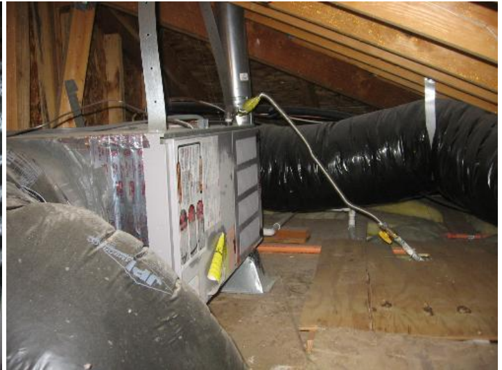
Heating Heater Condition
