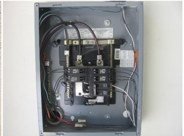
Electrical Sub Panel
