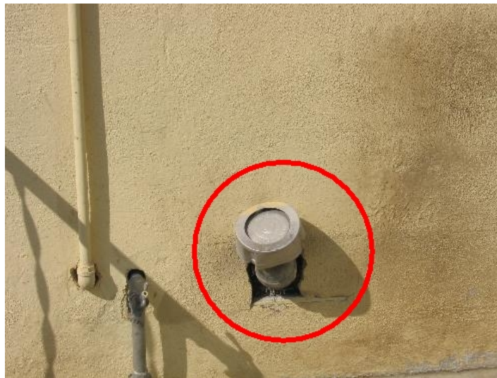
Improper installation of vent pipe. Exhaust vent from water heating in the basement area.
