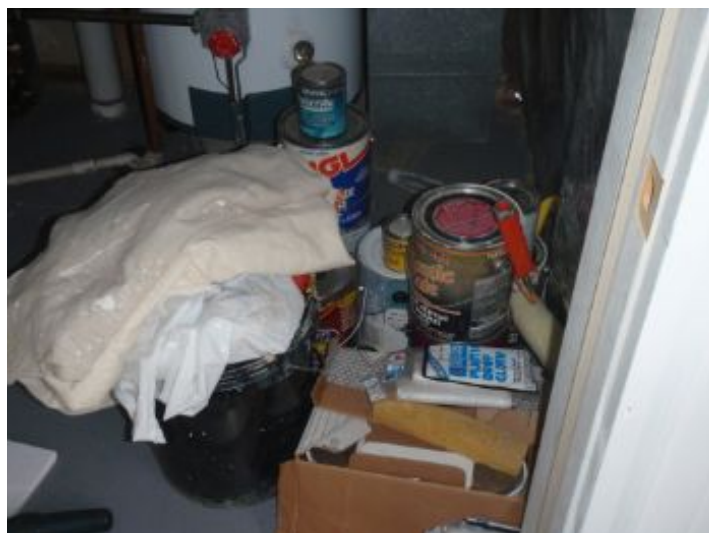
Combustible materials stored in furnace room.
