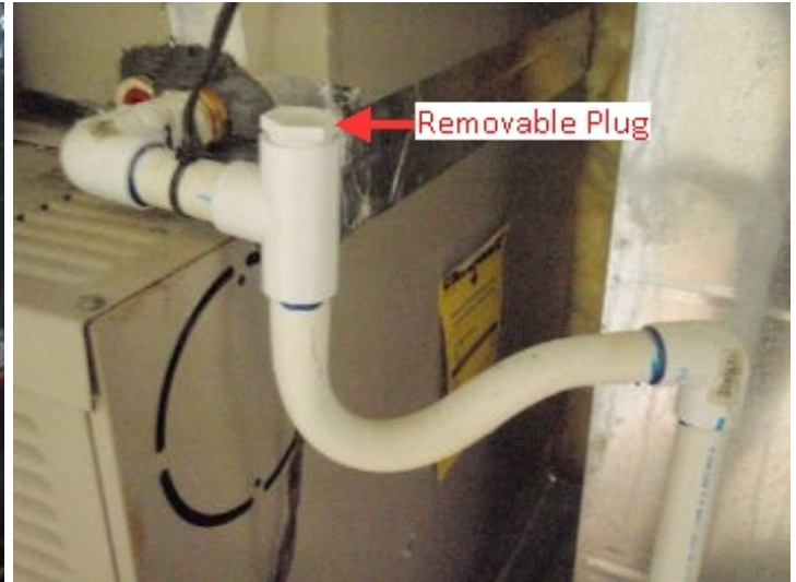
Example of a clean-out plug installed in condensate drain
