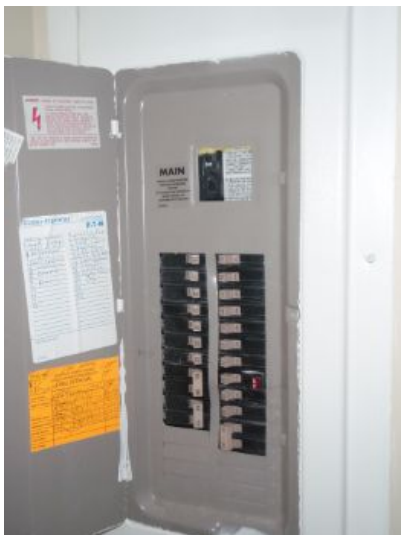
Cutler-Hammer brand electrical panel
