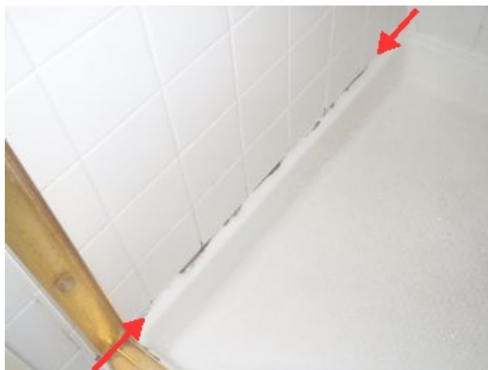
Caulking repair needed at master shower stall
