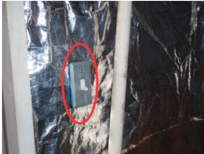
Furnace Electrical Safety Switch on Wall next to Furnace
