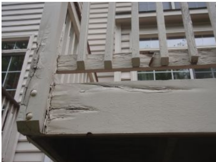
The deck perimeter trim board deteriorated and rotted
