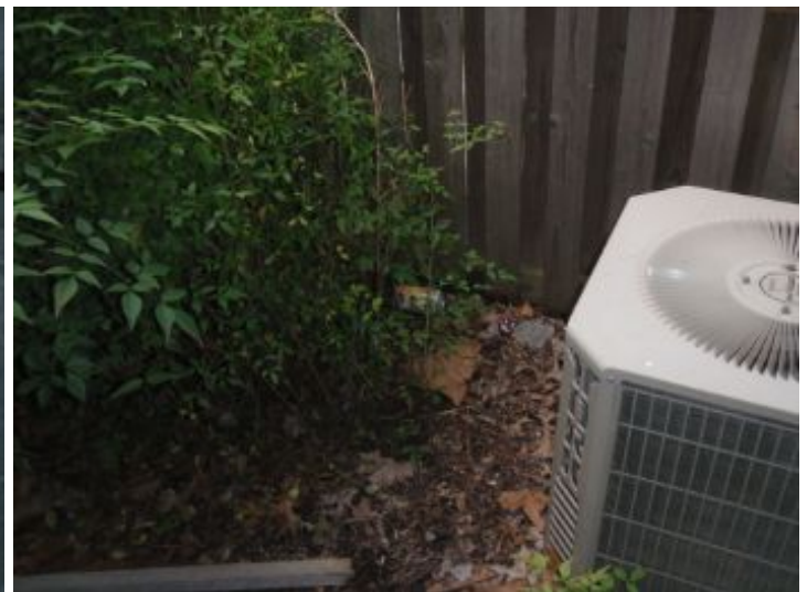
Vegetation needs pruning next to A/C Condenser
