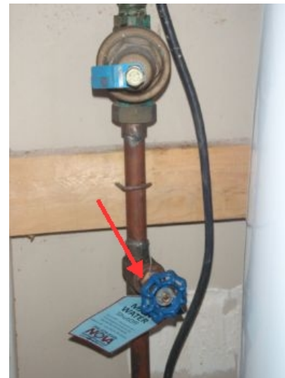
Main Water Shutoff
