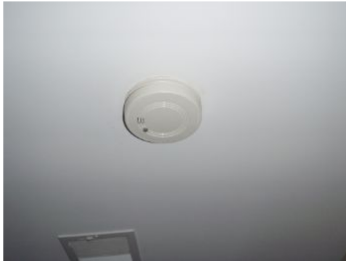
Smoke detectors in the house Inoperative
