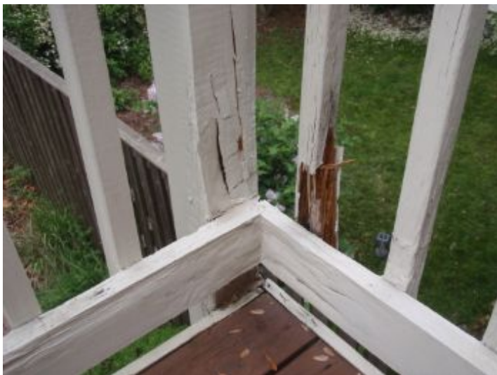
Several balusters are rotted and NOT SAFE
